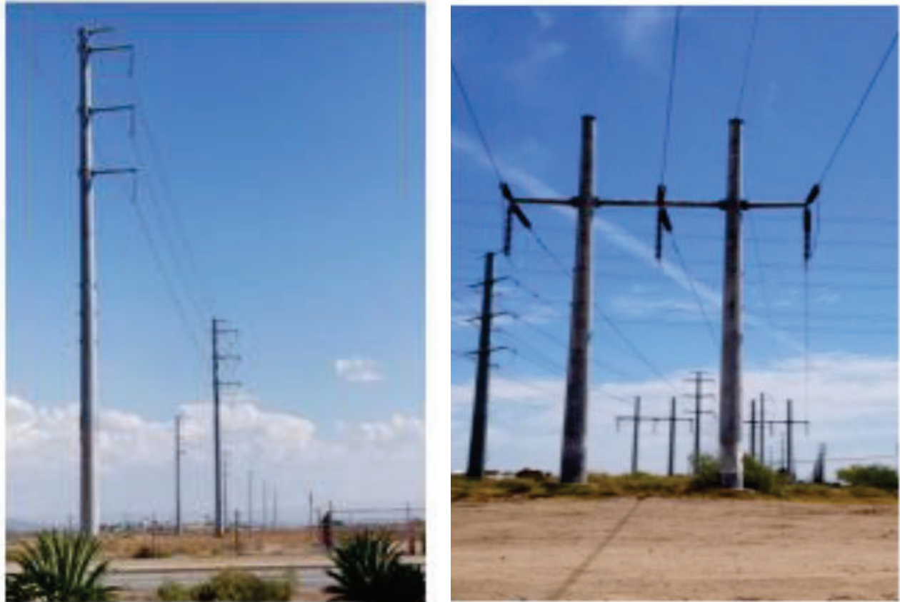
Figure 3. Typical 230-kilovolt Single-Circuit Monopole and Monopole H-Frame Designs
